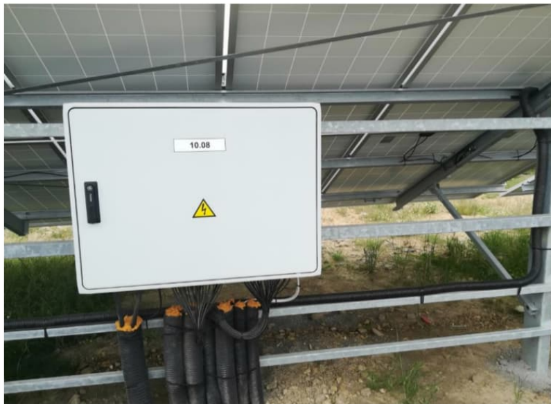
Plate 3-2. DC Electrical Box
