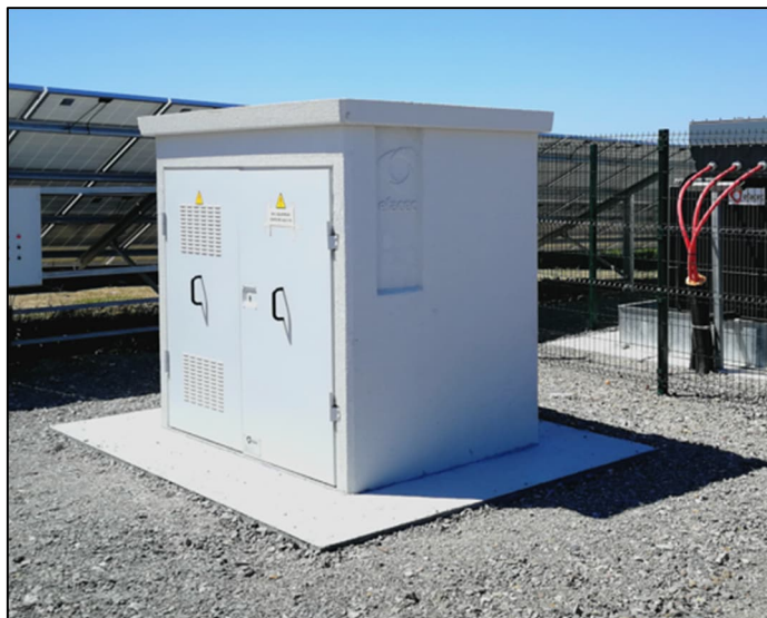
Plate 3-9. Outdoor cabin switchgear
