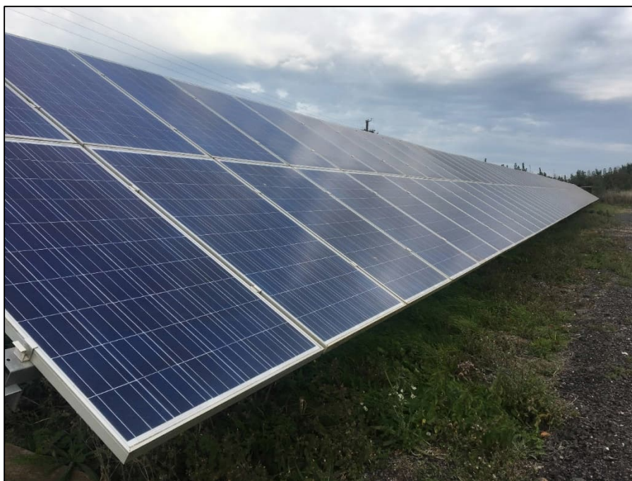
Plate 3-3. Solar panels (solar string) with south facing configuration
