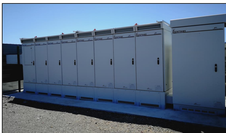
Plate 3-7. Typical outdoor centralised inverter
